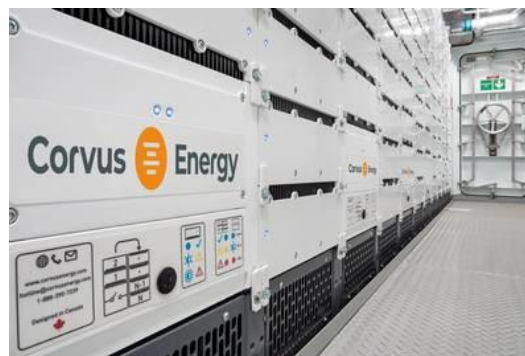
Figure 4 – “Corvus Energy” battery packs
